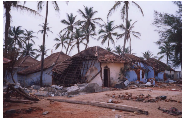
Damaged houses at Chinnavilai village.
